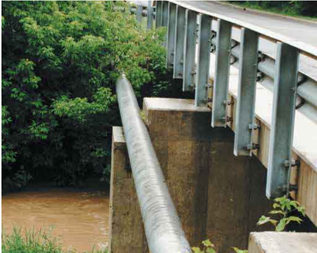
#2A Wax-Tape applied to bridge span, providing corrosion protection from road salt, physical damage and atmospheric corrosion.
