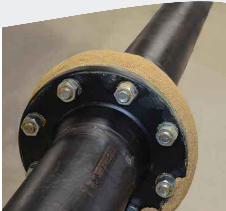
Fill-Pro PM-GP can be used to fill flanges prior to the application of Wax-Tape □ .
