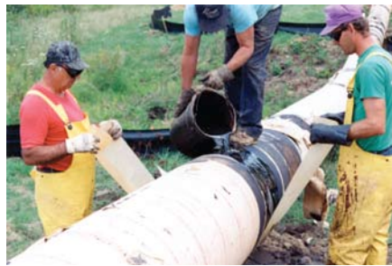
Innercoat wax coating being applied directly to the pipe surface using the Guard-Wrap wrapper as a "granny rag."
