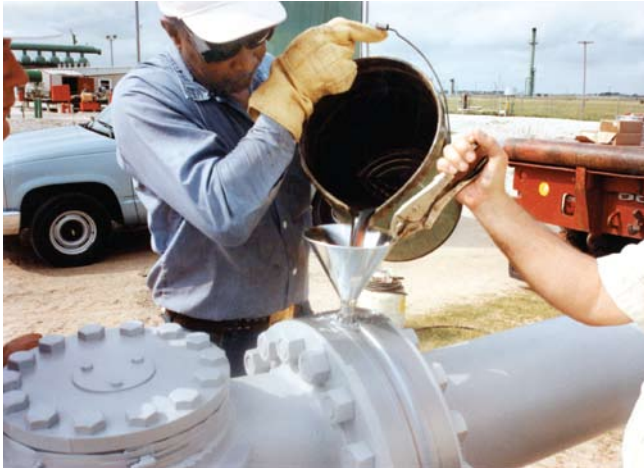
Flange filling is the process of pouring hot Innercoat between the flange faces to prevent corrosion.
