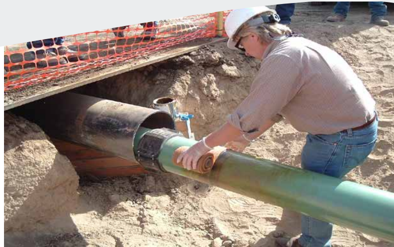
HT-3000 Wax-Tape does not require sandblasting. Here the tape is being applied to moderate-temperature pipe, but it can also be applied to hot in-service lines by using insulated gloves.
